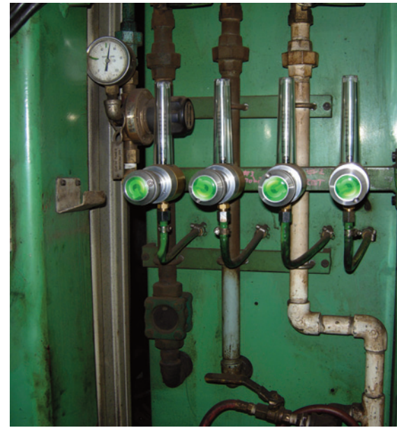
Figure 2 These gas regulators, integrated into a bulk distribution system, cause gas to flow in a consistent way around the arc, sources said. Photo courtesy of Syner-G Welding Regulators.
